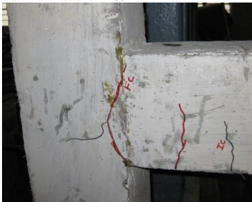
Figure.8 Failure Pattern of Conventional Concrete BC Joint
